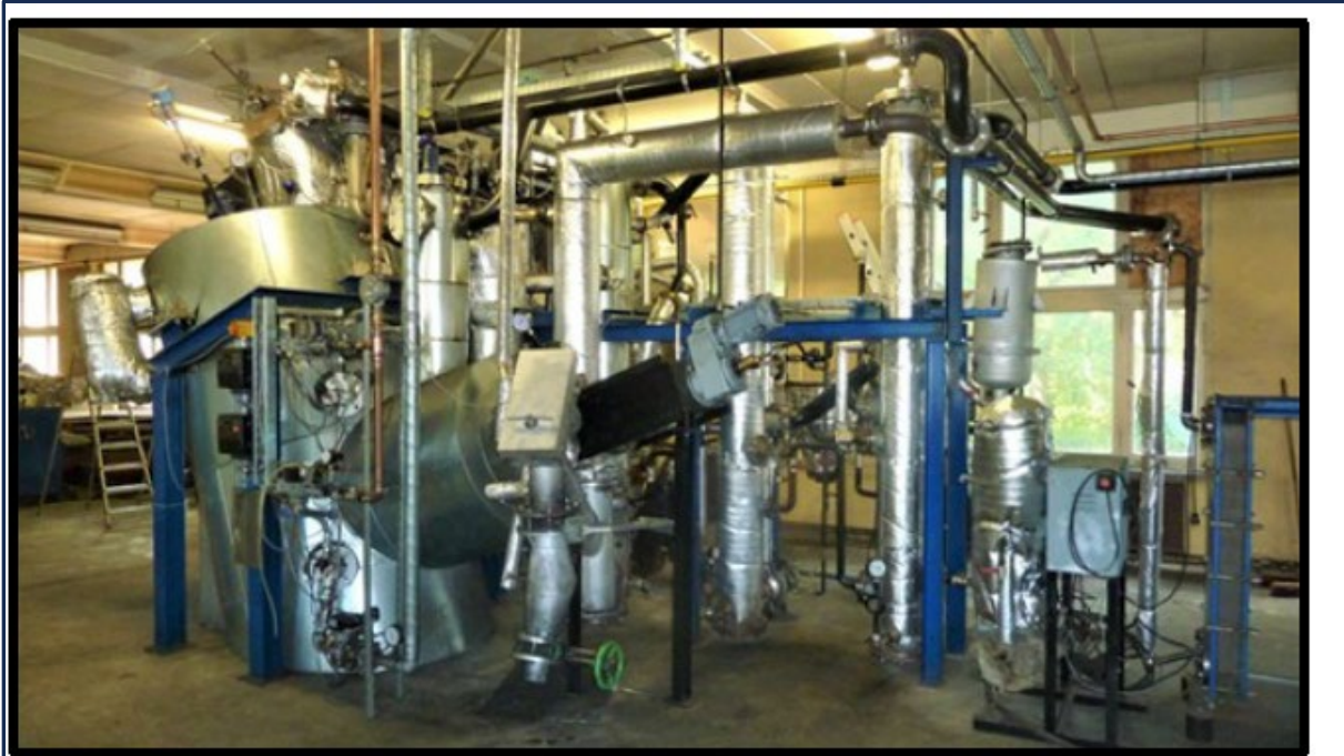
Figure 1. Photo of the pilot Thermolyzer™ line located in Forst, Germany
